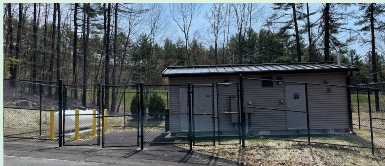
New Drummer Hill Pump Station constructed in 2021 pumps water up to the newly constructed 130,000 gallon Drummer Hill Tank.
